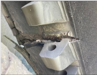
Part Defect Area Showing Adjacent Feature
