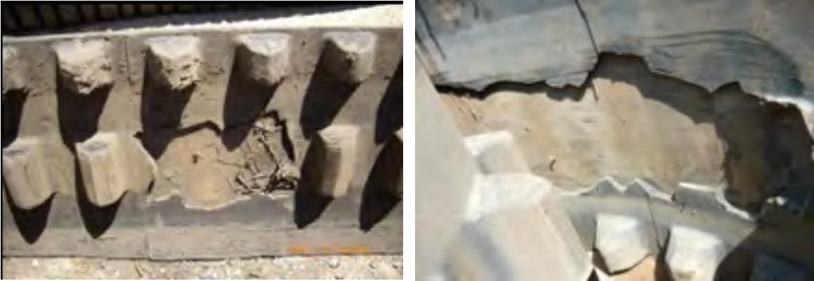
Drive Lug Loss (smooth separation)
