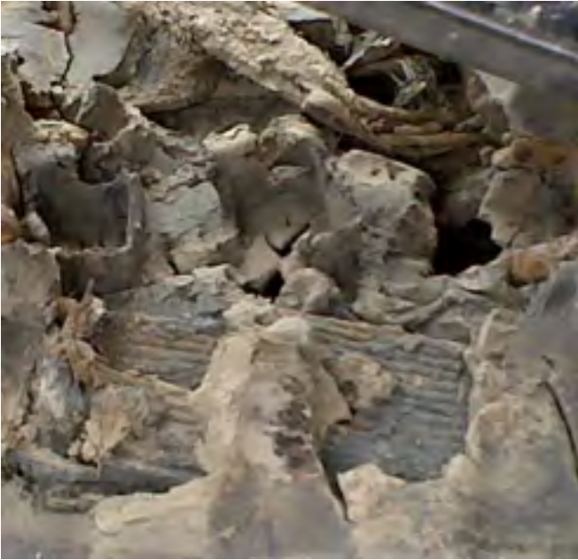
The shape of the rubber is ripped
