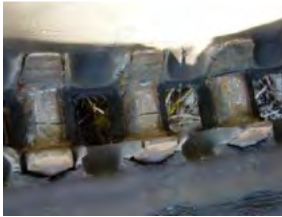
Drive bars cracks (impact)
